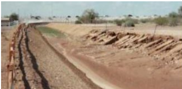
PROBLEM Severe erosion of ditch channel banks along roadway
